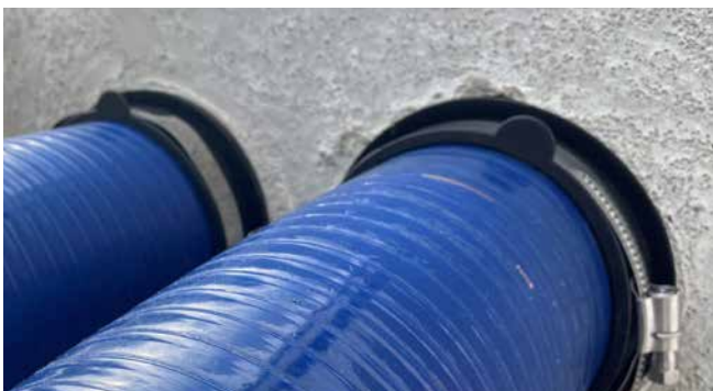
HSL150 KMA installed
