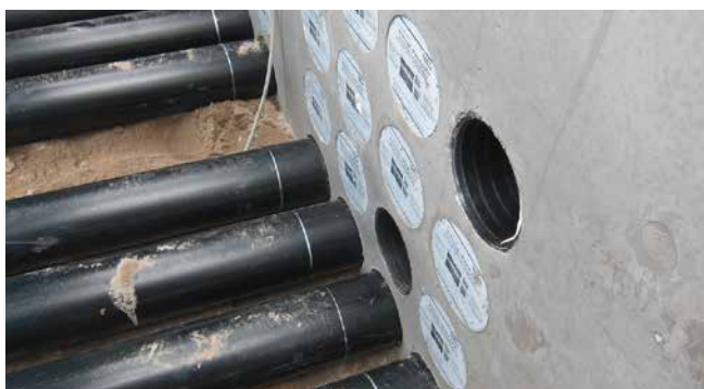
HSL150 GSM installed
