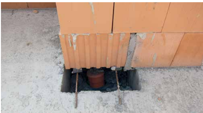
difficulty: retrofit gas-tight and vapour-proof sealing
