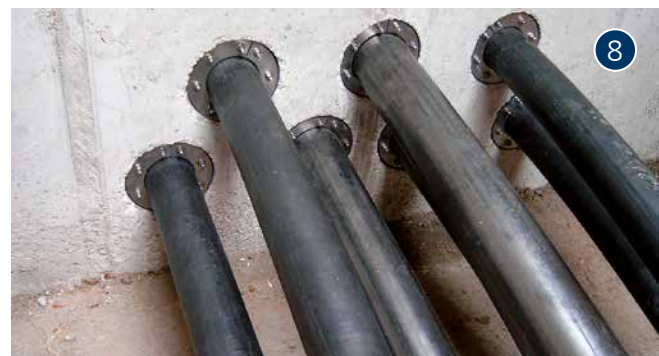
HRD press seals installed
