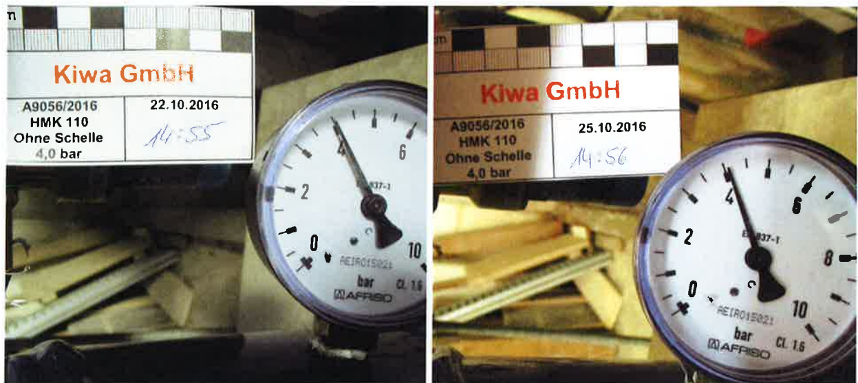
Figure A6. Water tightness test with the 4,0 bar water filled pressure bell (left: manometer on October 22 nd , 2016 at 2:44 pm; right: manometer after 3 days on October 25 th , 2016 at 2:56 pm).
