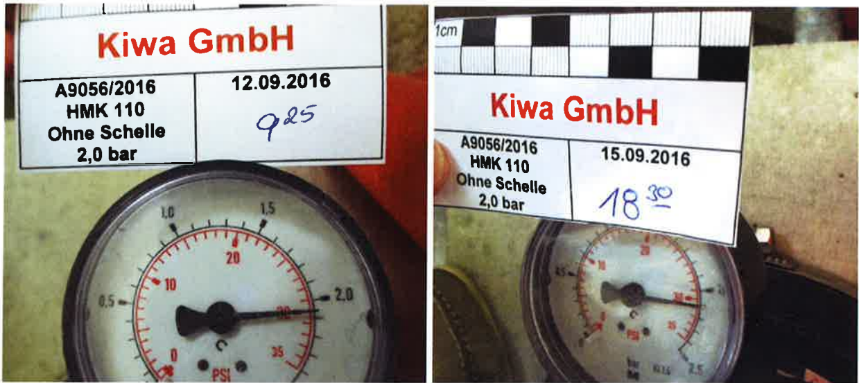
Figure A3. Water tightness test with the 2,0 bar water filled pressure bell (left: manometer on September 12 th , 2016 at 9:25 am; right: manometer after 3 days on September 15 th , 2016 at 6:30 pm).
