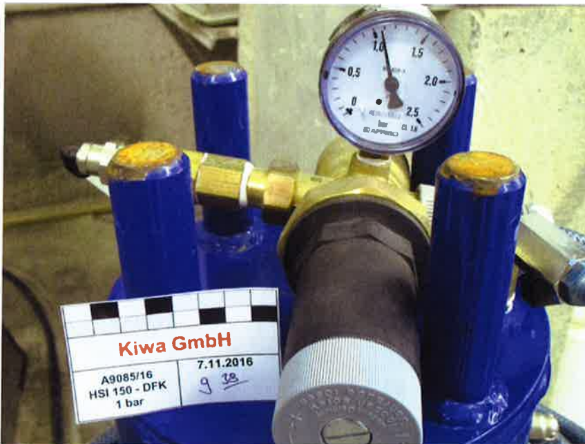
Figure A1. Water tightness test with the \geq 1,0 bar water filled pressure bell (manometer at the beginning of testing on November 7 th , 2016 at 9:38 am).
