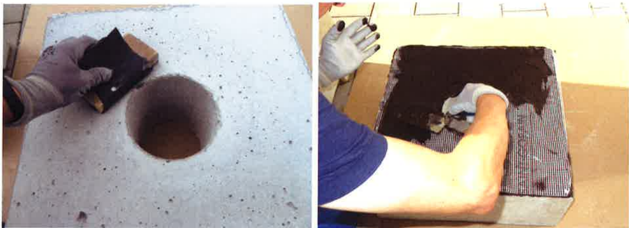
Figure 2. Leveling of the uncast concrete surface (left) and applying of the polymer-enhanced bituminous thick-coat system (right).
