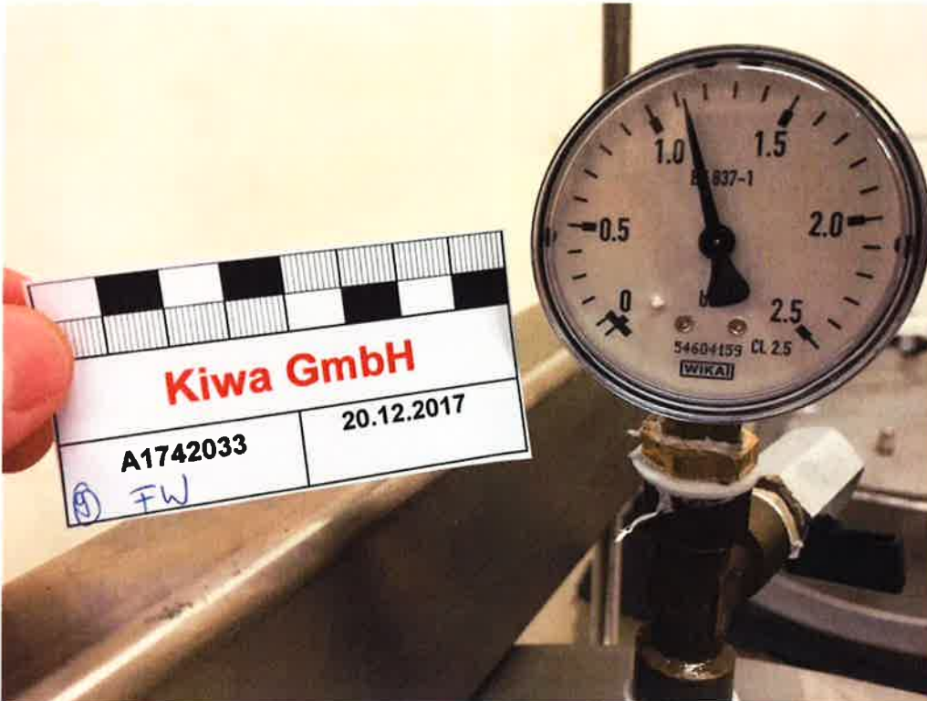
Figure A1. Water tightness test with \geq 1,0 bar water filled test cylinder (manometer at the beginning of testing on 20.12.2017).
