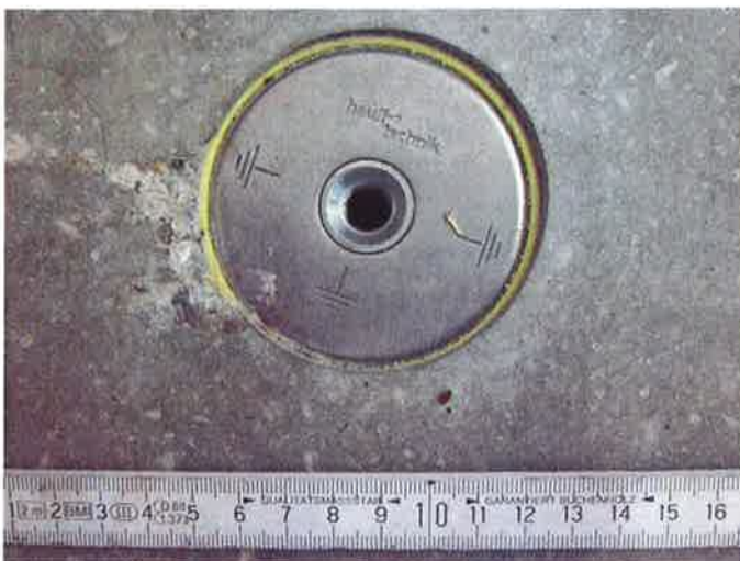
Illustration 2: Grounding penetration passage HEA-IS-M12/100, concrete trough inner side
