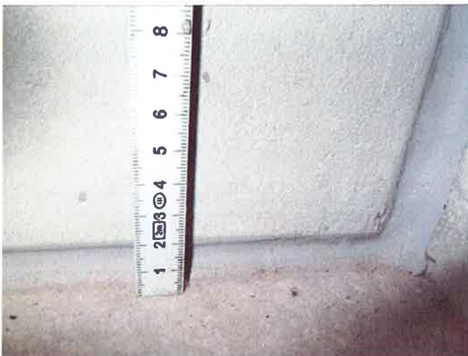
Illustration 26: Sealing joint Sikaflex Tank N on the side facing the oil after 92 days
