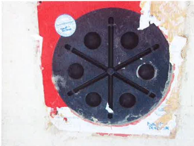
Illustration 23: HSI 150 K2-100 with close-off HSI 150-D (2 nd experiment), trough under-side after 92 days
