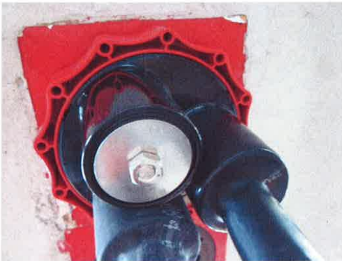
Illustration 20: HSI 150 D3/58 with seal plugs VS58/60, hot and cold shrink-on sleeve in HSI 150-K 100, trough under-side after 92 days
