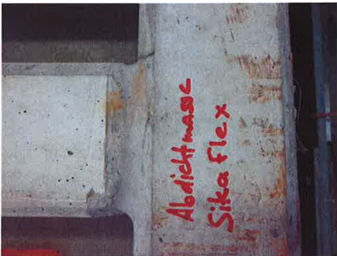
Illustration 9: Transverse bulkhead sealed with sealant mass Sikaflex Tank N (side view and top view)
