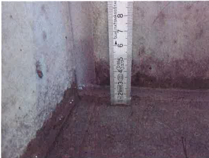
Illustration 13: Oil level in the trough immediately after the insertion of the oil in the area of the sealing joint (approx. 15 mm)
