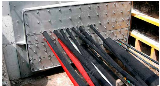
split rectangular flange with multiple cables
