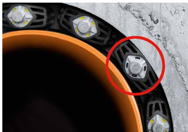
GKD with one segment not tightened – installation error immediately detected.
