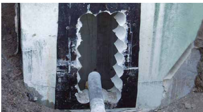
high-voltage cables and ducts have to be subsequently sealed in the shaft wall
