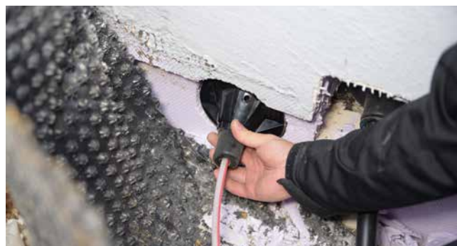
GFH20 PRO installé
