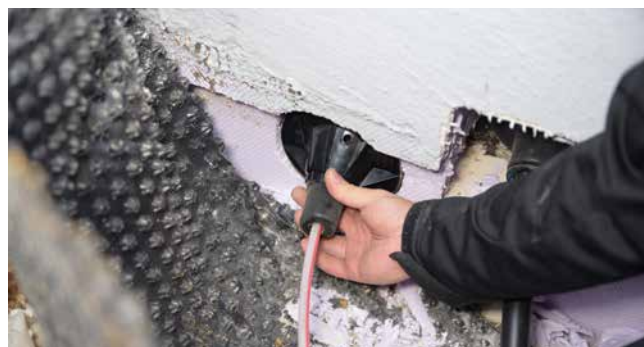
GFH20 PRO installé
