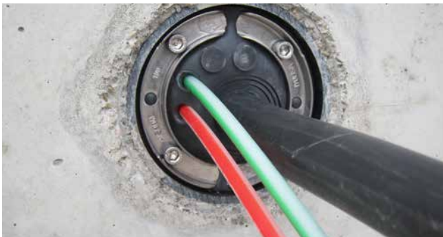
HSD100 EW installé
