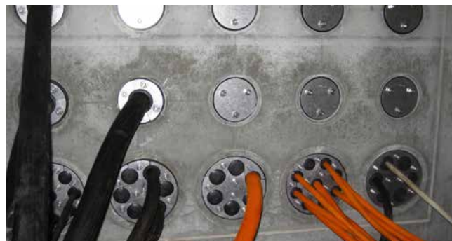
HRD150 SG installed in fibre cement wall sleeves
