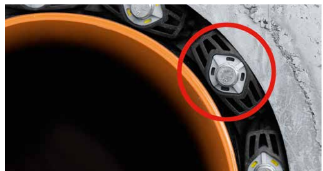
GKD with one segment not tightened - installation error imcarriertely detected.
