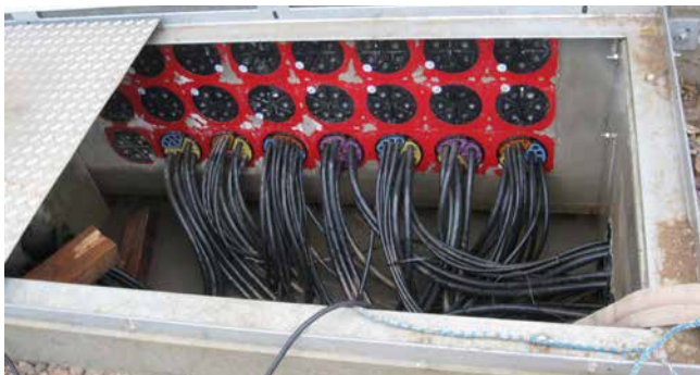
HSI150 - wall inserts fitted with SEGMENTO sealing for control cables in a transformer house
