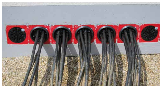
low-voltage cables sealed with HSI150 DG 6x10-36
