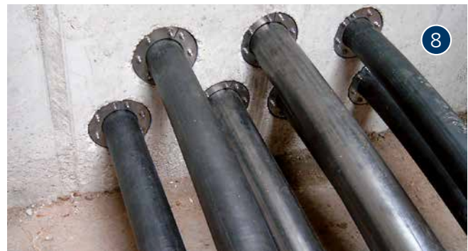
HRD press seals installed
