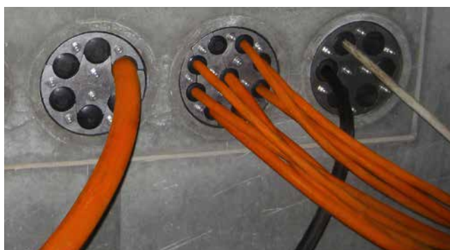
HRD150 SG installed in fibre cement wall sleeves
