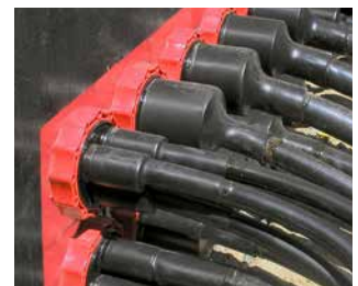
station entry: low-voltage cable sealed HSI90 D1x75 WS and HSI90 D3x32 WS
