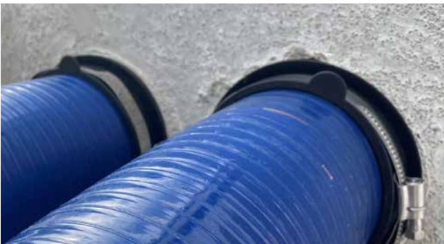
HSI150 KMA installed
