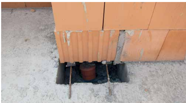
difficulty: retrofit gas-tight and vapour-proof sealing
